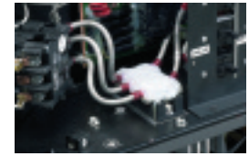
Coated Electrical Connections
